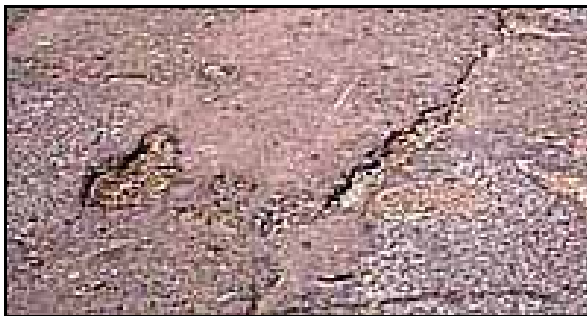
Not so much a pothole as a crater
